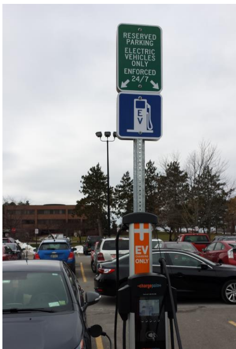
Figure 16: Charging Station in “D” lot.
