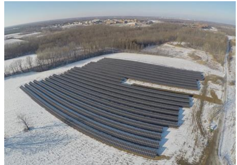
Figure 13: RIT 2 MW solar array
